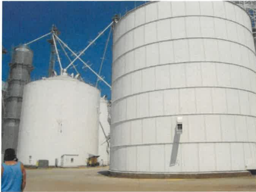
Figure 4: Welded-Seam Silo (Left) May Be Watertight; Bolted-Plate Silo (Right) Is Not Watertight
