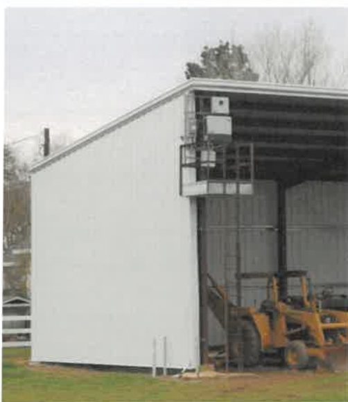
Figure 24: Elevated Electric Service and Equipment
